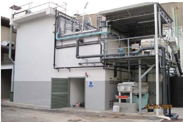
▲ Outdoor UASB reactor in Food Processing Plant, Shah Alam
