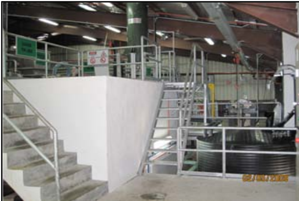
▲ Indoor UASB reactor in Food Processing Plant, Subang Jaya
