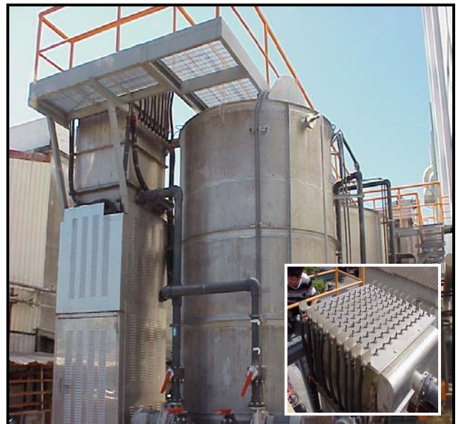
▲ Fered-Fenton reactor of a PCB plant
