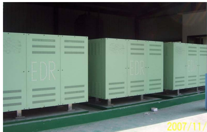
▲ EDR system in wastewater treatment plant
